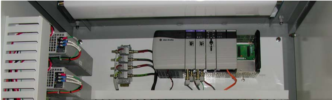
The above picture is the mounted HPI Allen Bradley Control Logix Controller.
