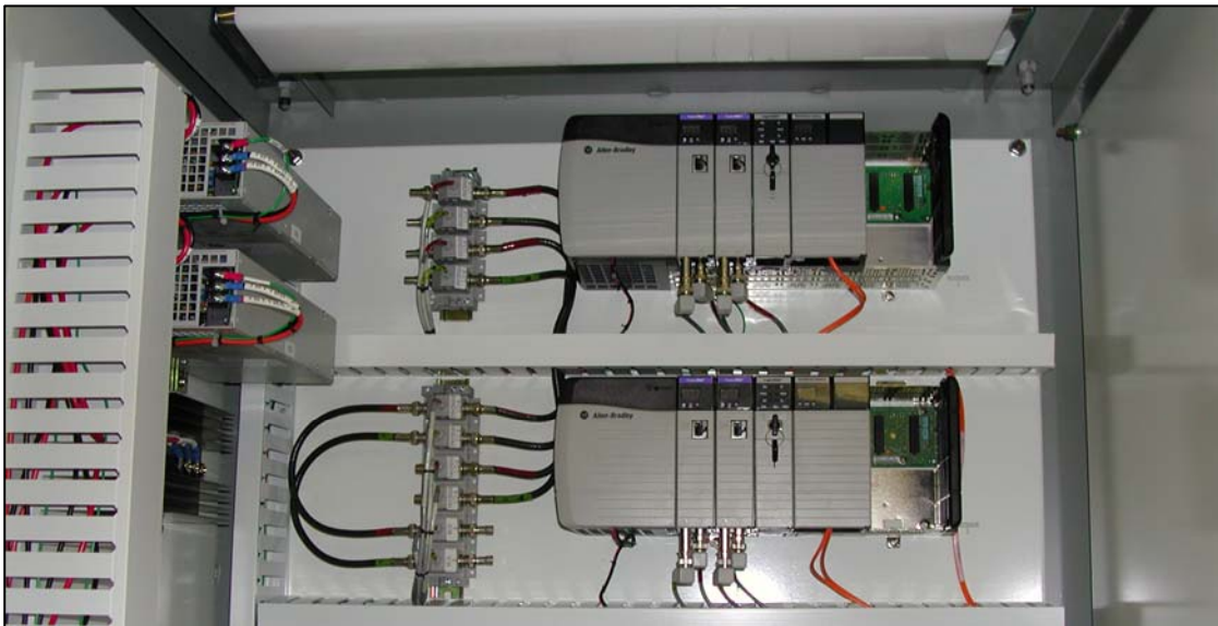
HPI Dual Redundant ControlLogix Installation
